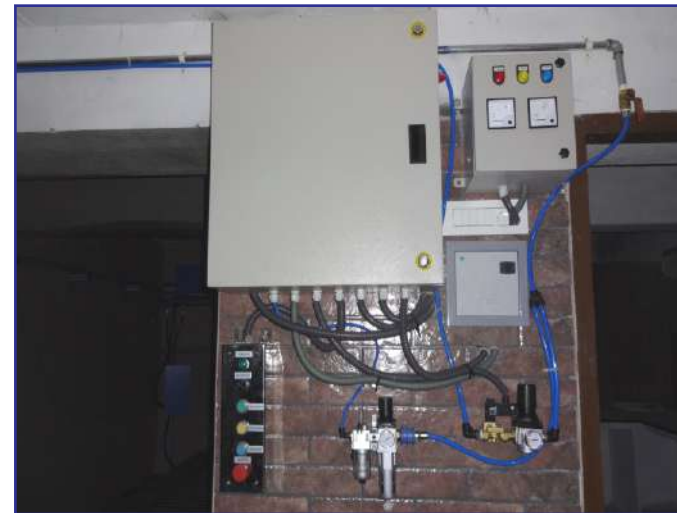
Main Control Panels
